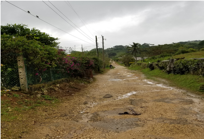
Epworth Main Road, St. Ann, before JSIF's intervention.
