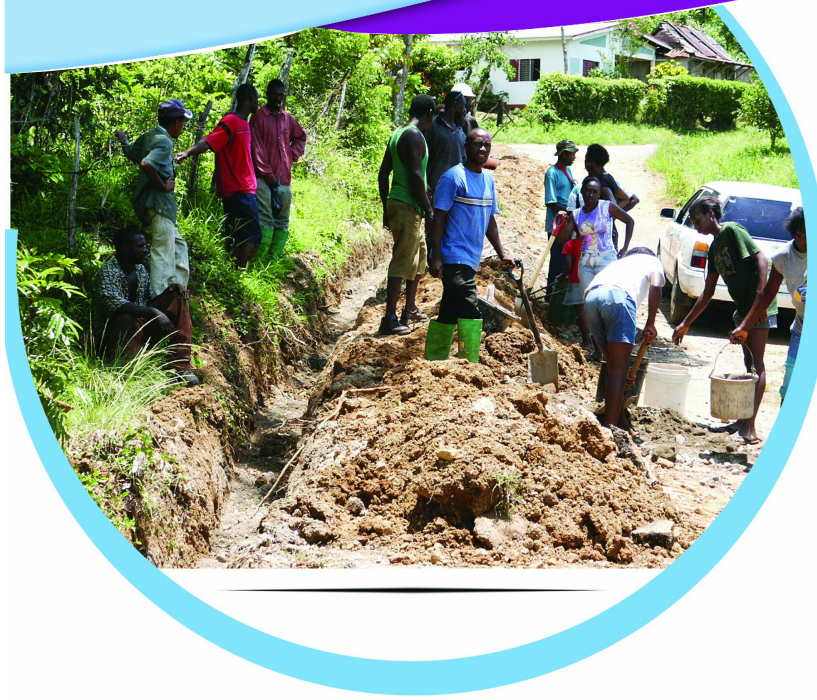
Mountain Pass community labourers digging the trench to lay pipe for the water supply system
