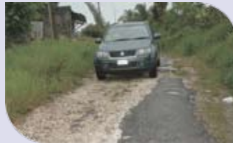
The existing Accompong road that is to be rehabilitated through funding from the Government of Jamaica.
