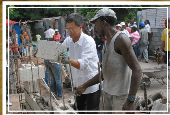
Minh Pham (left), Resident Representative of the United Nations Development Programme in Jamaica, is assisted in laying blocks by a labourer in the Whitfield community in St. Andrew during a zinc fence removal and replacement work day in the community.
